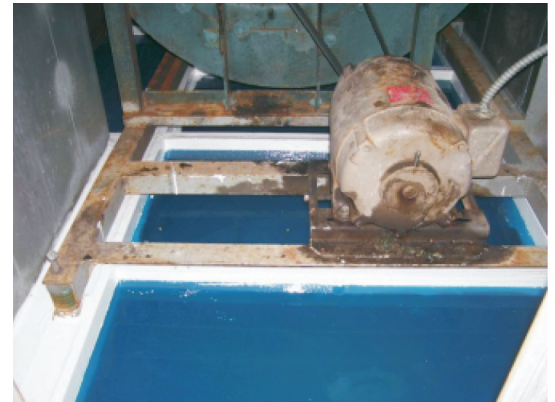
A Rusted HVAC Pan treated with Panshield
