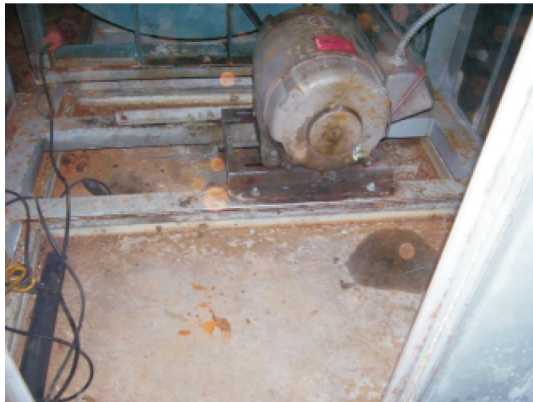
A Rusted HVAC Pan
