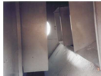
Rusted vertical walls in air handling unit coated with V570
